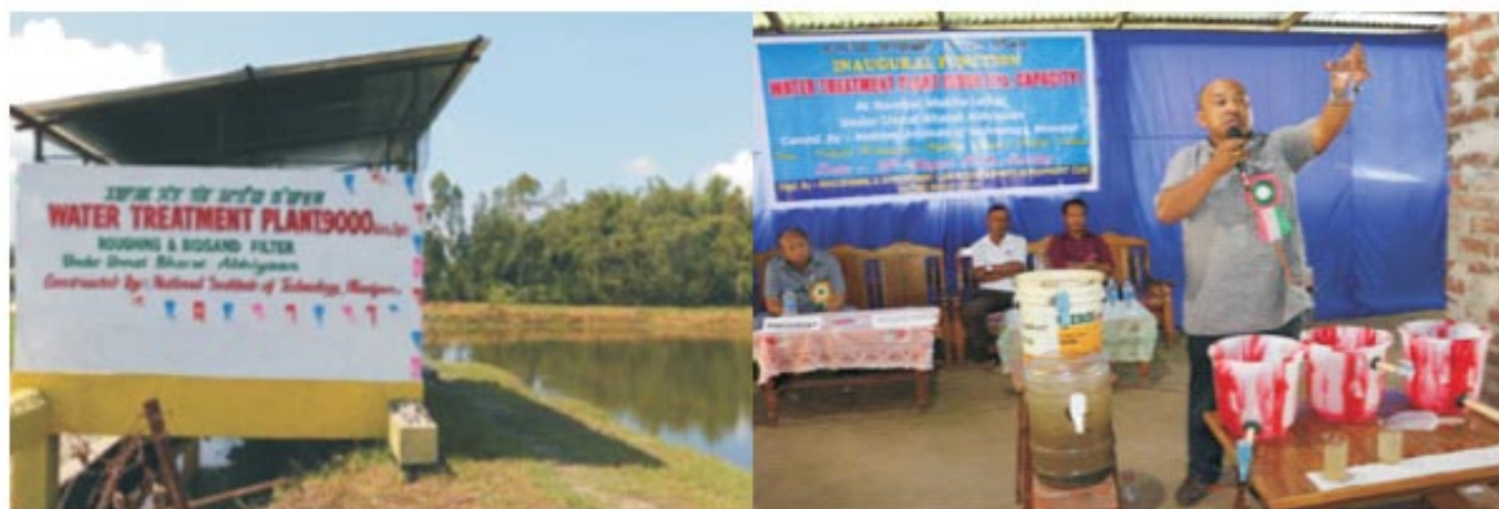
Figure 8: (i). The Pond & Water Treatment Plant (ii) UBA Coordinator, NIT Manipur (Dr. P Albino) giving awareness on operation and maintenance of the Treatment plant community-based BIOSAND Filter
