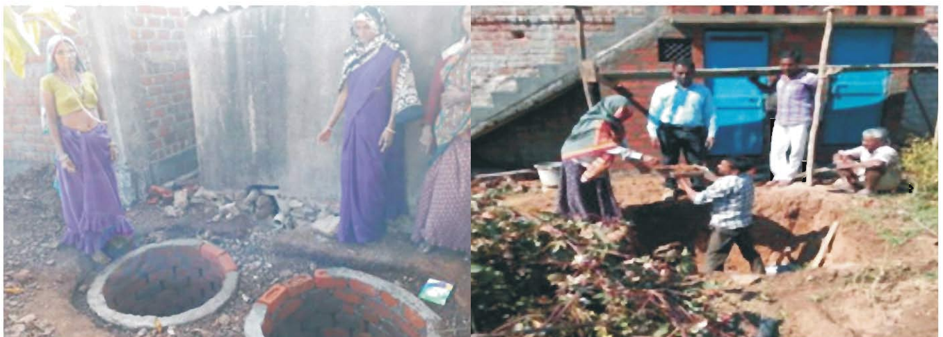
Figure 6: Laying out of dimension for toilet construction and initiating digging of Twin-pit
